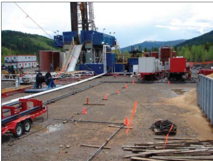
Managed pressure drilling equipment at the Nikanassin wellsite included a Weatherford IIP 1000 rotating control device (RCD; Fig. 6)
